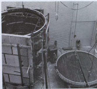
Figure 4. HIFOD Chamber Cold-wall prior to installation.
