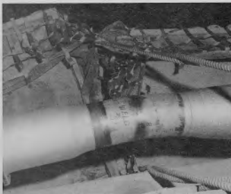
FIGURE 37 - INVAR WELD IN VJ PIPING ON A MOBILE LAUNCHER MARKED UP FOR X-RAY INSPECTION
