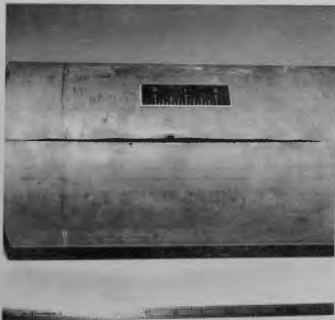
FIGURE 32 - SECTION OF DAMAGED INVAR PIPE
