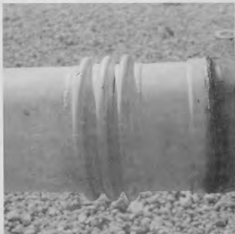
FIGURE 29 - FATIGUE CRACK IN THE CONVOLUTE OF AN EXPANSION BELLOWS IN A VJ PIPE
