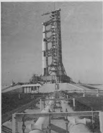
FIGURE 27 - VACUUM JACKETED PIPING INSTALLED IN A CROSS COUNTRY RUN AT A LAUNCH SITE
