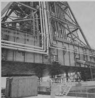
FIGURE 28 - VACUUM JACKETED PIPING INSTALLED AT THE BASE OF A MOBILE LAUNCHER
