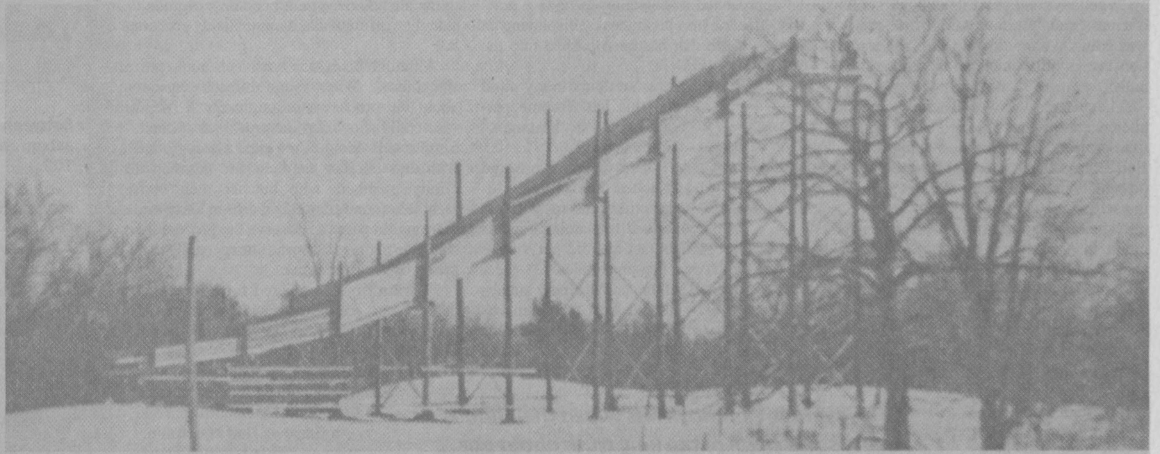
January 17, 1963 • The Maine Campus During Christmas Vacation members of the ski team built a new, 25 meter jump for training purposes. Smaller than the old structure it is 115 feet long and 40 feet high. The jump's outrun slopes uphill so that the jumper can easily stop and ski back to the base.
