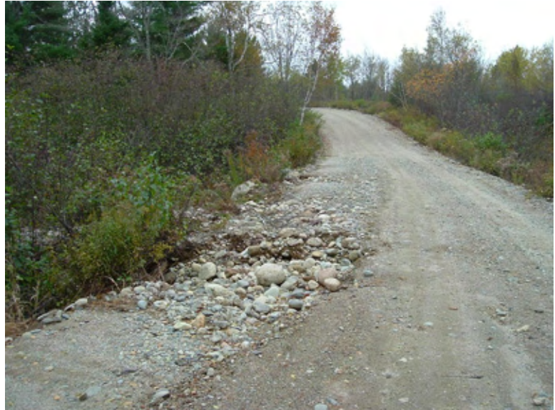
A washed out camp road. (T. Gamache)
