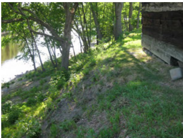
View of the eroding slope behind the Block House. The slope should be stabilized to stop erosion, improve riparian habitat, and protect the historic resources.
