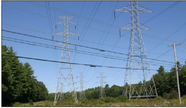
Figure 2-36 The visual impact of the utility lines is increased because they are set against the sky.
