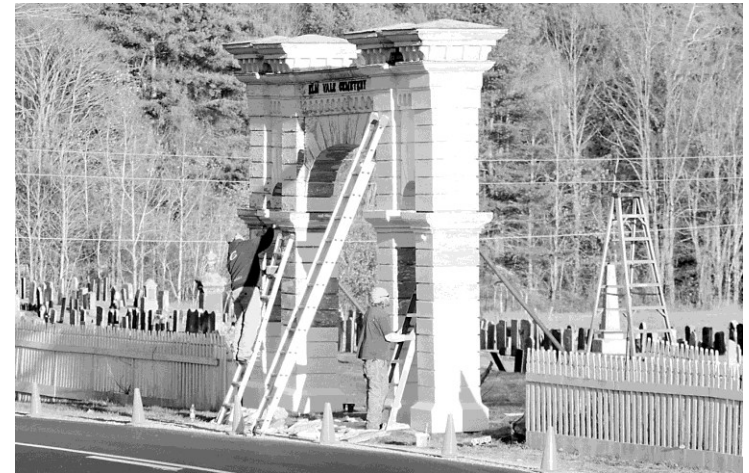
Restoration of the Elm Vale Cemetery arch is nearly done. Work will be completed in the spring.
