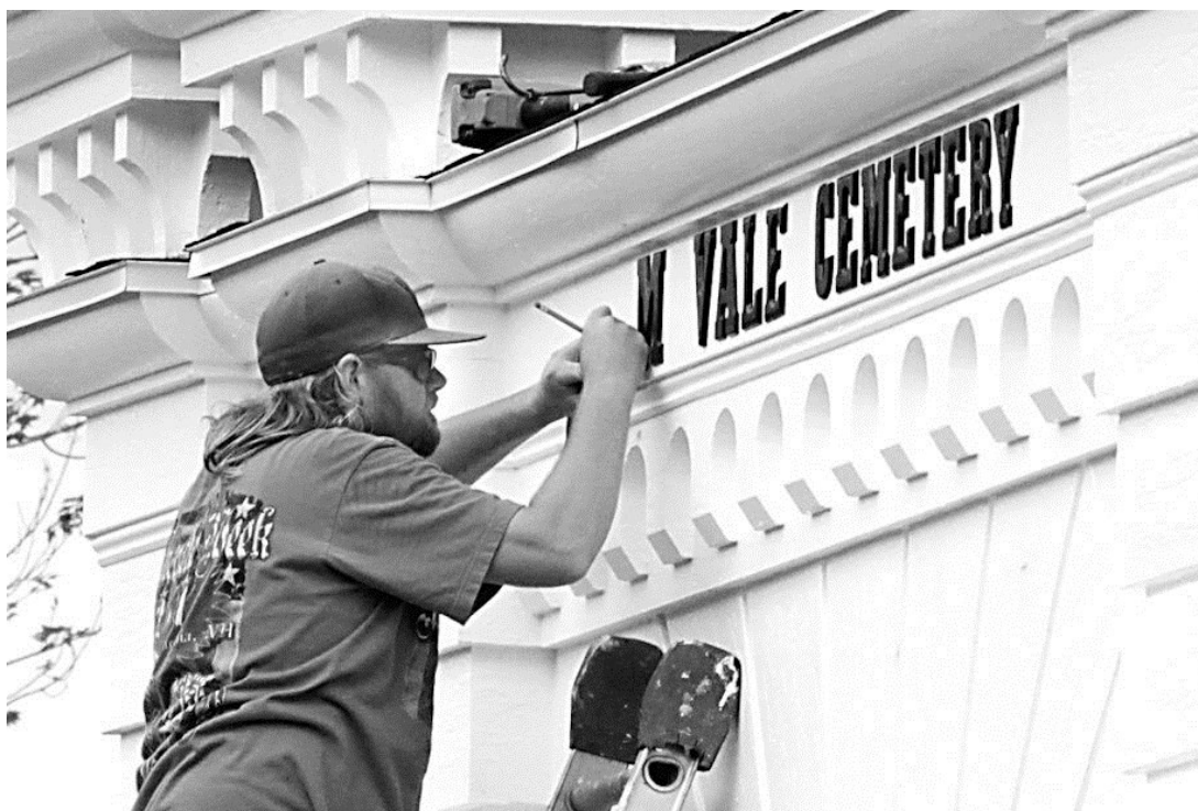
ELM VALE CEMETERY ARCHES - Justin Grover is shown attaching the lettering for Elm Vale Cemetery in August, signaling the completion of the arch rebuilding project by PDJ Construction of Waterford. The historic arch restoration was funded entirely from donations. A new fundraising campaign will begin this spring to restore the easterly archway.
