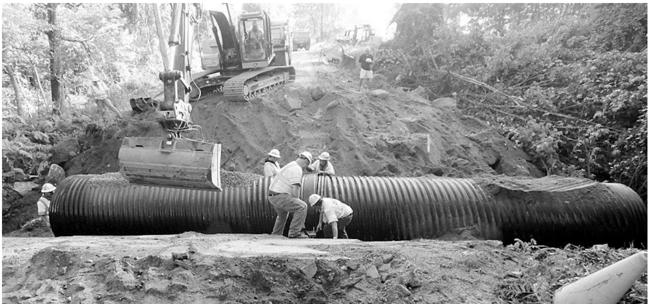
EMERGENCY REPAIR - Maine Department of Transportation crews worked until dark on Thursday, Sept. 17, and throughout Friday replacing the defective old box style stone culvert on Sweden Road. A sinkhole opened up in the road requiring the state to undertake immediate emergency repair measures. The road was shut down for two days, reopening early Friday evening. The disturbed strip of highway was paved on Monday, Sept. 21.
