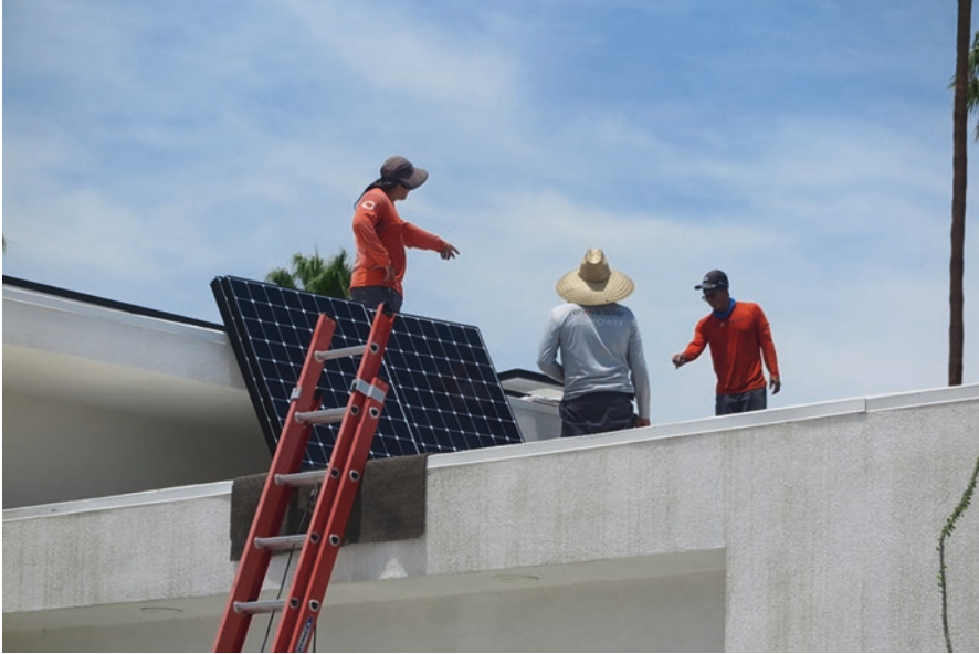
Fig. 7.1 Semi-skilled solar installers on a roof installing solar panels, Palm Springs, CA
