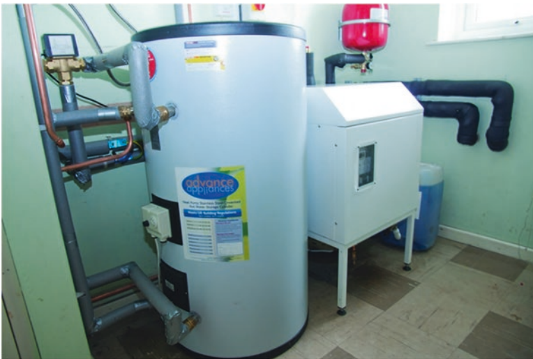
Fig. 2.13 Ground source heat pump inside a home (Source: Yorkshire Housing)
