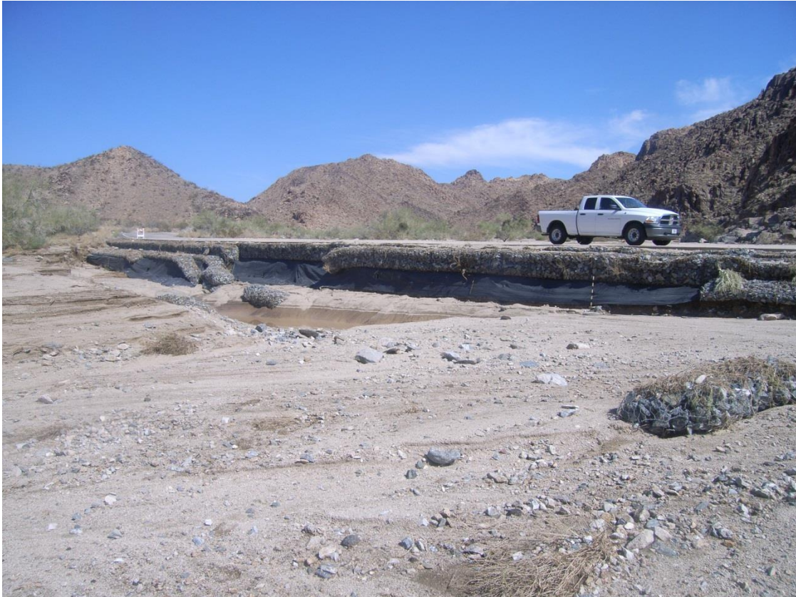
Figure 6.15: Southern road damage location. The area adjacent to the road was scoured out by the runoff during the September 13, 2011 event. Courtesy the National Park Service.
