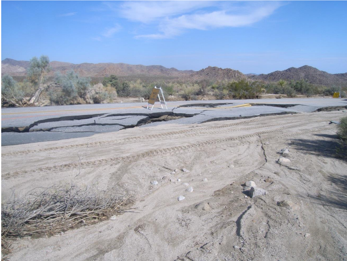
Figure 6.14: Northern road damage resulting from runoff on September 13, 2011. Courtesy the National Park Service.
