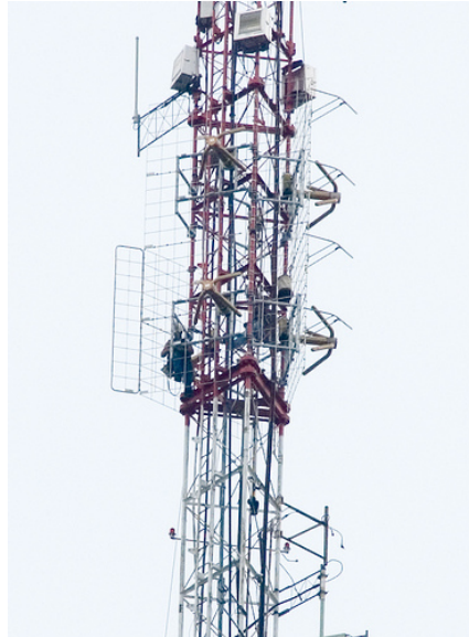
Figure 3.8. The arrangement of transmitters on a tower (Logan, 2007)
