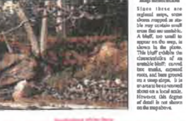
Bluff face showing vertical erosion. This photograph shows a typical bluff face with vertical erosion. The bluff is composed of unconsolidated sedimentary rocks, such as sandstone, siltstone, shale, and claystone. The vertical erosion is caused by the action of waves and wind. The bluff face is steep and vertical, and is often found along the coast of Maine.
