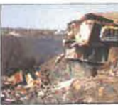
Bluff face showing erosion and a building nearby. This photograph shows a bluff face with significant erosion. A building is visible in the foreground, illustrating the potential hazard of bluff erosion to property.
