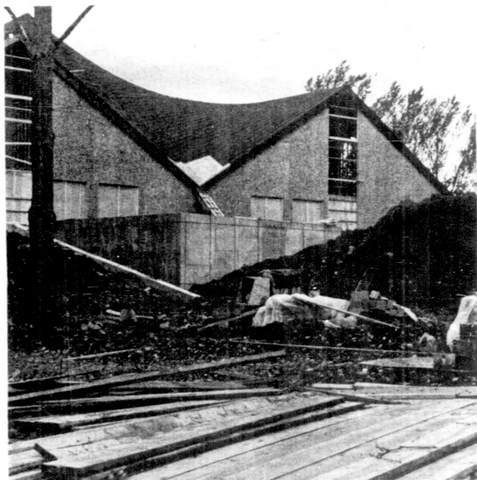
BESIDES CONTENDING with progressively colder weather, workmen at the Alfond Arena will have to pay closer attention to their materials. Eight hundred dollars worth of construction materials has been stolen from the site so far. Photo by Russ McKnight
