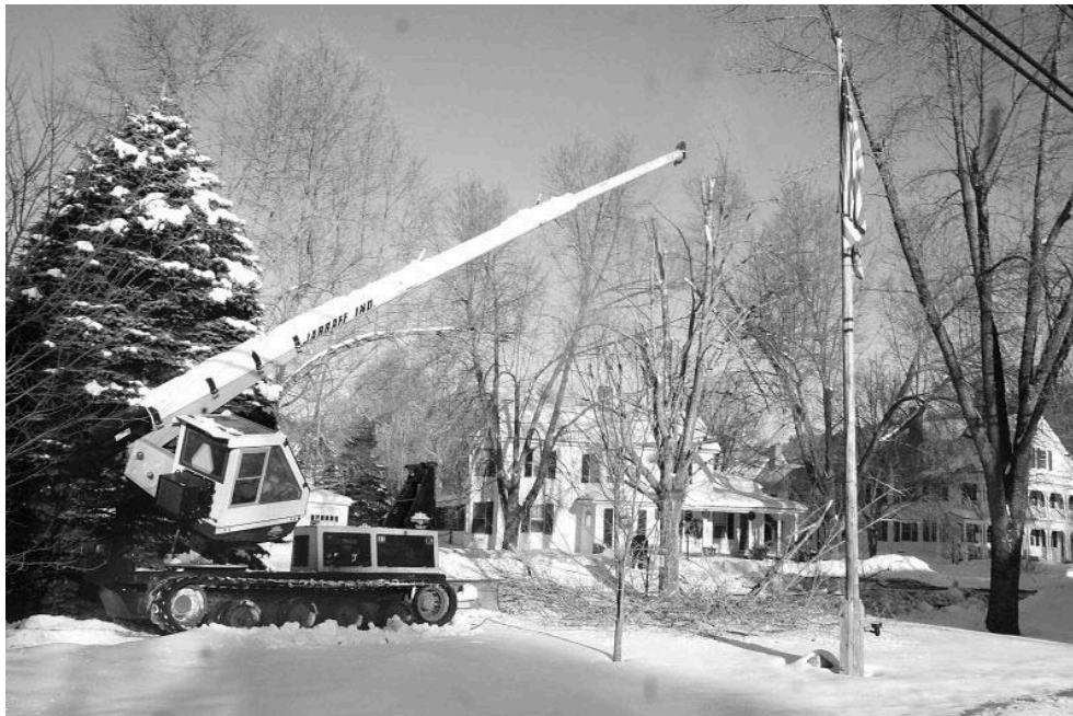
Todd Sawyer of TRS and Sheldon Rice of Rice Tree Service donated their time and equipment to remove two dying maple trees on the Waterford Common. Here, Todd operates his Jarraffe to trim the upper branches before Sheldon cut the trunk. Disease-resistant elms will be planted in the spring.
