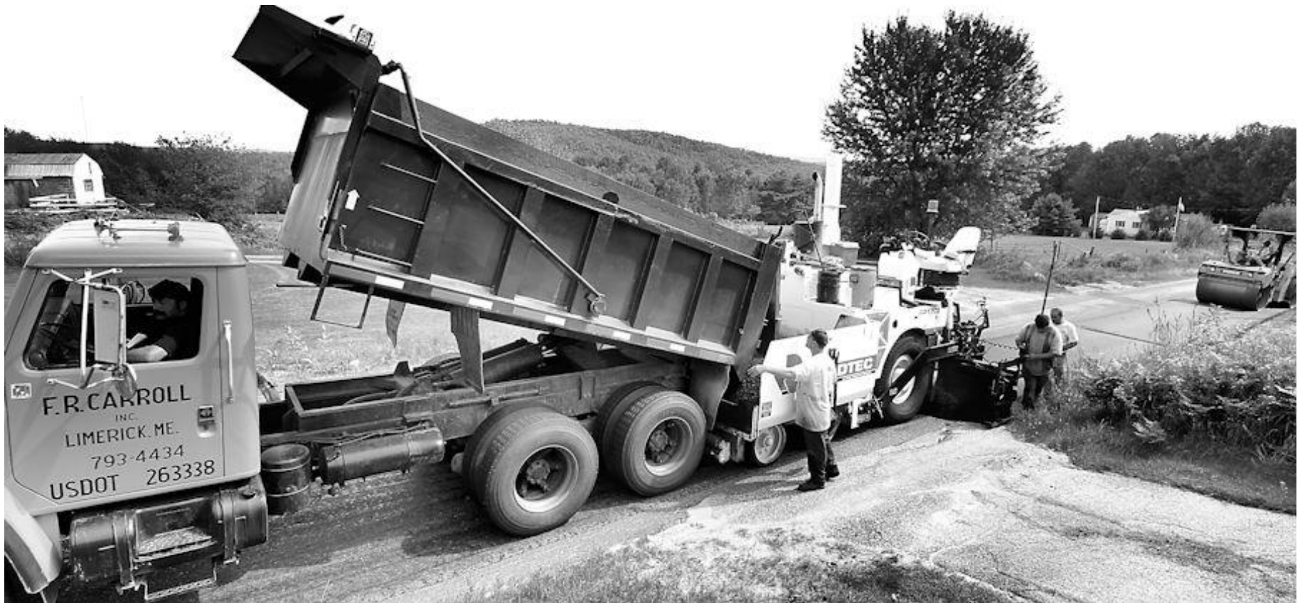
A crew from F.R. Carroll paved Blackguard Road Sept. 9 covering 8,500 feet using 1,400 tons with 21 trucks hauling from Limerick
