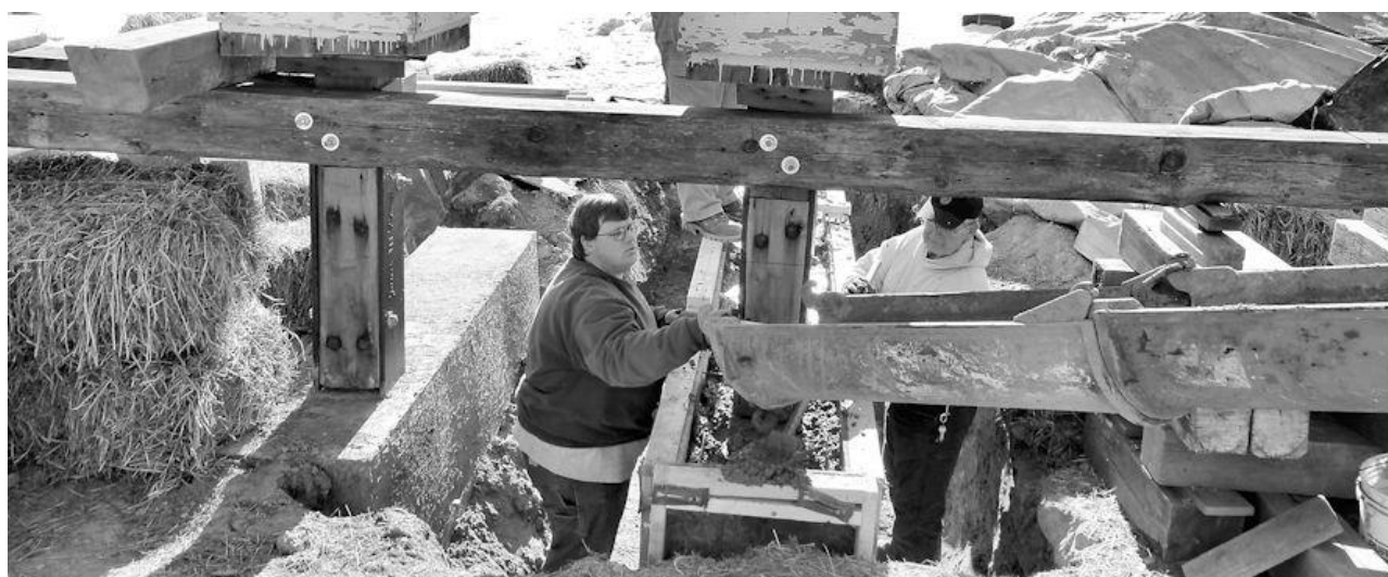
James Long and sons poured concrete Feb. 10 for one of two outside supports under the westerly gate. The first pour on the two inside supports was done Jan. 26, seen on the next page.
