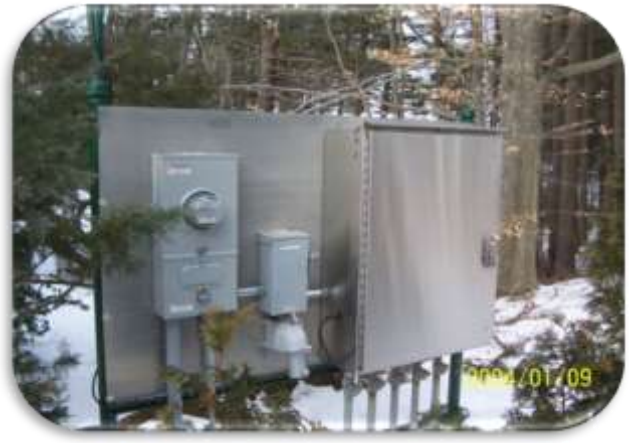
Glenhaven Pump Station
