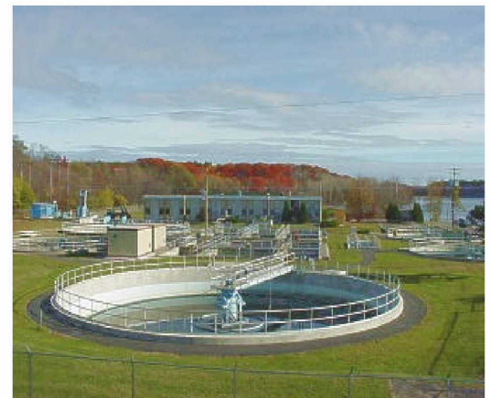
Saco Waste Water Treatment Facility
