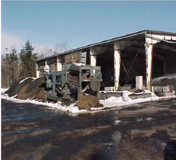
Old Orchard Beach Aerated Static Pile Compost Facility continues to treat wastewater treatment plant sludge from Saco since 1986.
