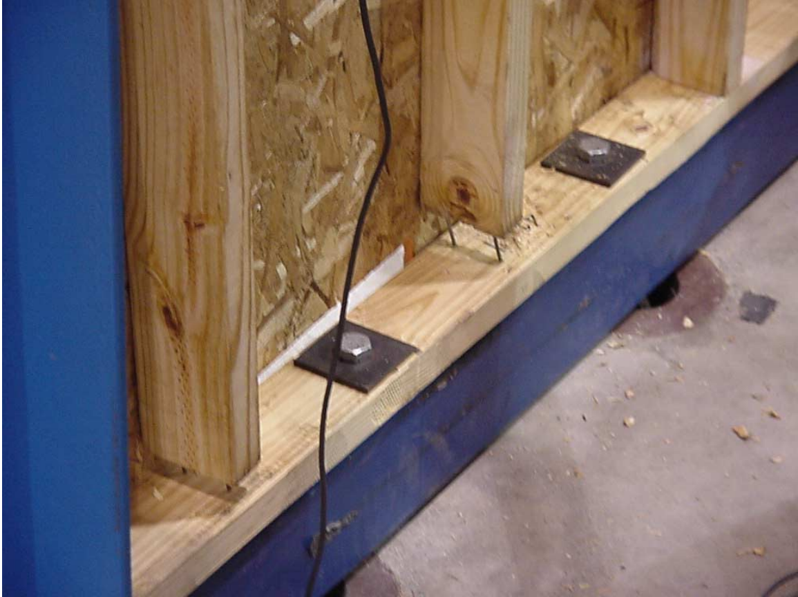
Figure 5.7 Shear Wall Base Bolts.
