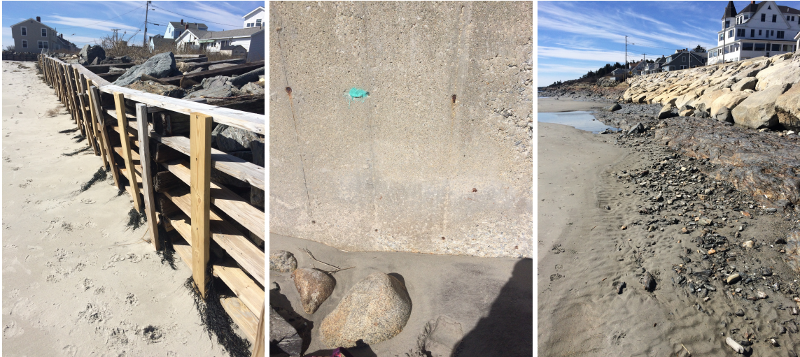
Figure 8. Different types of seawalls present at Higgins Beach. From left to right, wooden ballasted with stone at HI03, concrete at HI02, and riprap atop bedrock at HI01 (DeVoe, 2016b).
