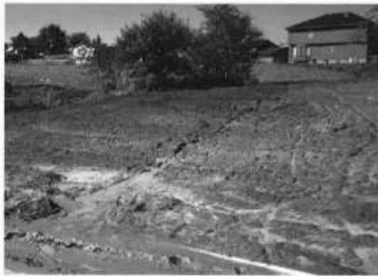
In this suburban neighborhood, sediments were washed into the street by the rain, because the soil was not protected during house construction.
