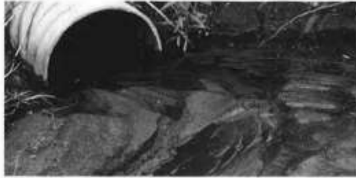
Sediments have filled up the opening of this drainage pipe that empties a stream into a lake.
