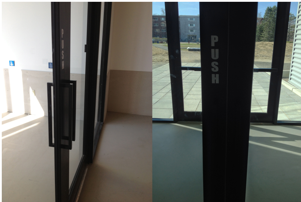
Figure 4. Example of a poorly designed door here at the University of Maine
