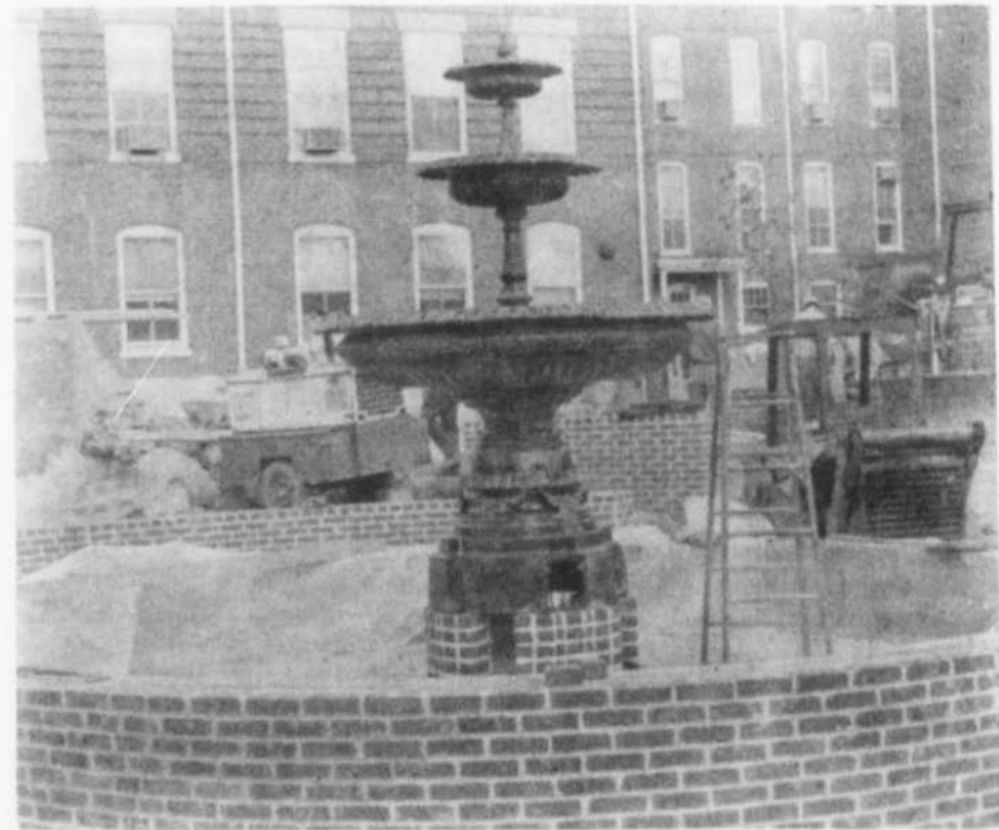
The placing of the fountain on Wednesday, brought the mall project one step closer to completion. The entire project is expected to be finished Dec. 15th.
