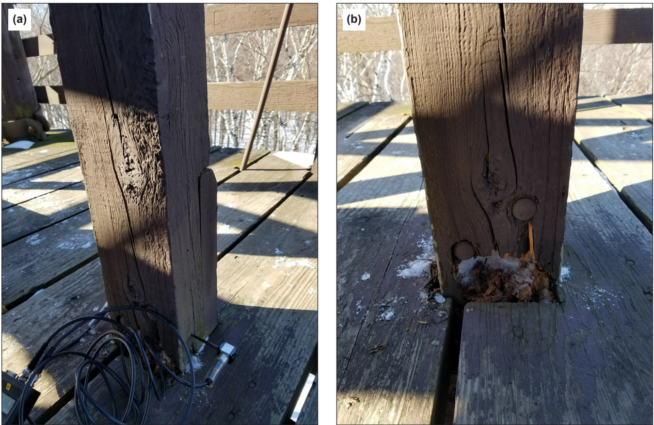
Figure 7. Central stairway support at platform 2. (a) Stress wave timing measurement showed significantly high readings (426 \mu s, equivalent to 853 \mu s/ft), indicating severe decay. (b) Visible deteriorated wood.
