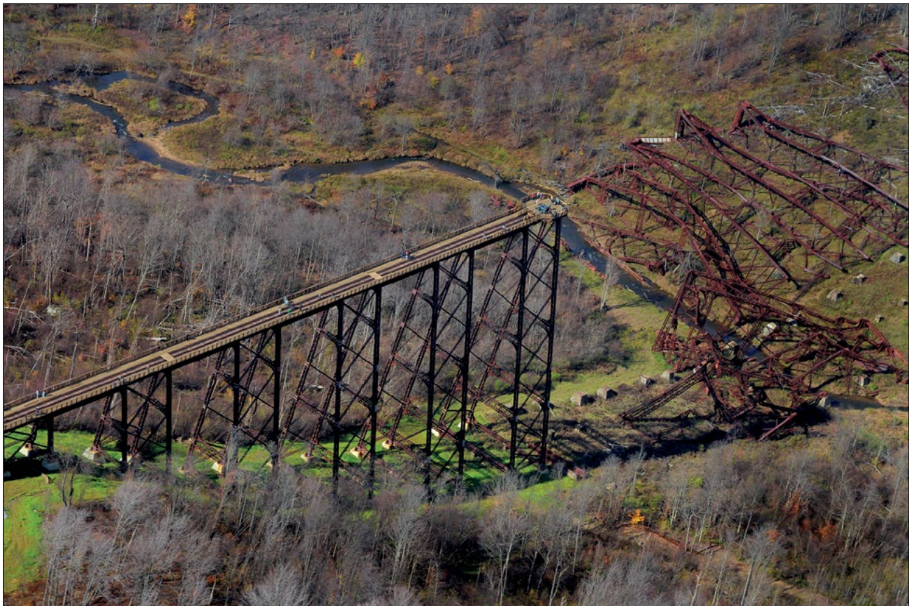
Kinzua Bridge in McKean County, Pennsylvania. This landmark was heavily damaged by a tornado in 2003. Photo by Greg Czarnecki, Pennsylvania Department of Conservation and Natural Resources, used with permission.
