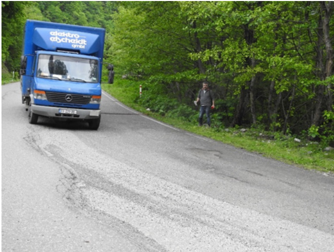
Figure 17: Road subsidence, evidence of Khoko landslide (2)
