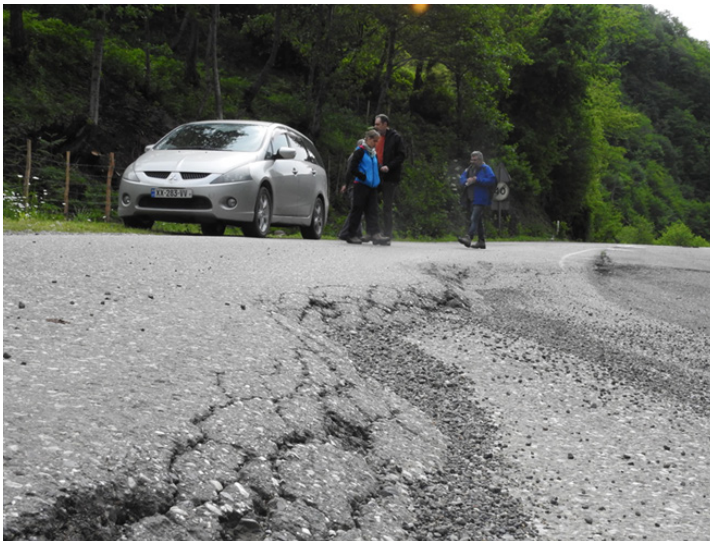
Figure 16: Road subsidence, evidence of Khoko landslide (1)
