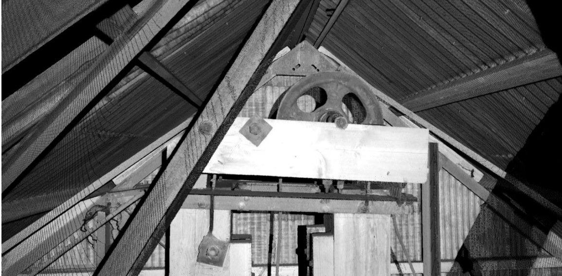
Figure 3.8. Point cloud image from HDS7000 laser scanner. Drop Hammer pulley and bridgework. (Image exported from Leica Cyclone 7 software).
