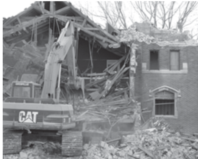
The original American Reformed Church, which became Northwestern's Playhouse in 1970, was razed in December.
