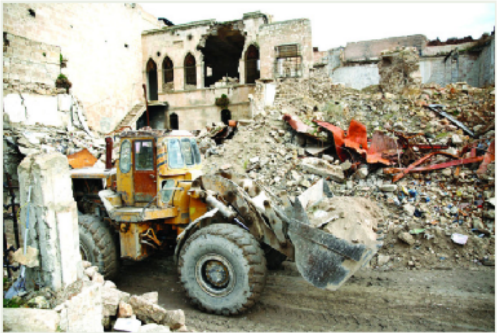
A bulldozer removes rubble from damage of the old market in the old city of Aleppo, Syria. (AP)
