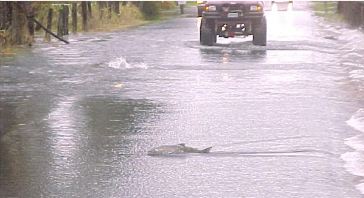
Figure 12: A salmon swimming upstream using its “nose” and traveling on top of the road because the culvert underneath is clogged with debris (NOAA, 2017).
