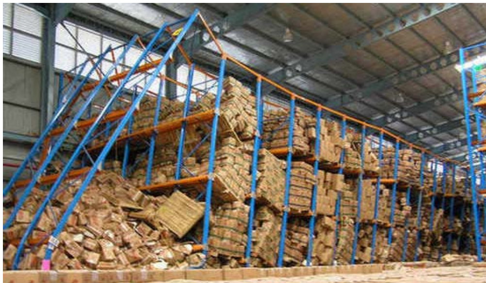
Figure 3.4: Series failure of racking systems in warehouses [29].
