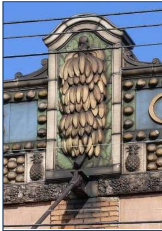
Above photo of the was taken in 2009 by the Cleveland Landmark Commission prior to being
