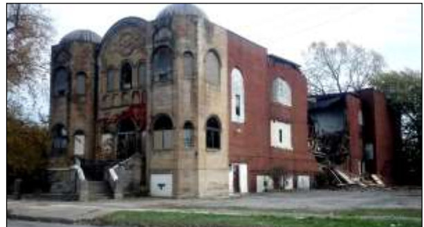
Photo taken November 4 th 2013. The building was demolished within a few days Photo taken by Jeff Morris
