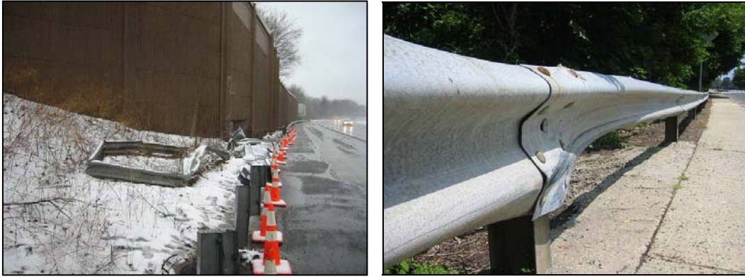
Figure 1. Does the damage to these w-beam barriers hinder their performance?
