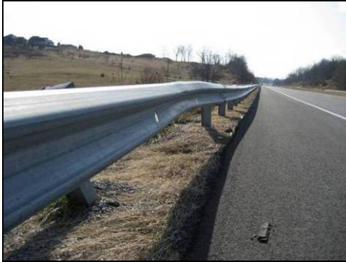
Fig. 1. Minor damage to a strong post w-beam barrier on a major state route.
