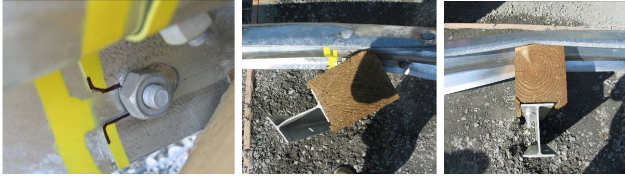
Fig. 16. Test 07-4: Detail view of splice bolt damage after test (left) and post damage at splice (center) and non-splice location (right)
