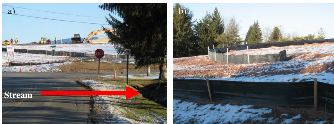
Figure 32: (a) Upstream construction site between Smoketown Road and Beagle Club Road. (b) Construction site with sediment guards.
