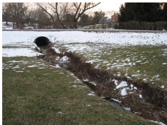
Figure 34: Highly eroded banks along the upstream reach of Miller Run (west of U.S. Highway 15).
