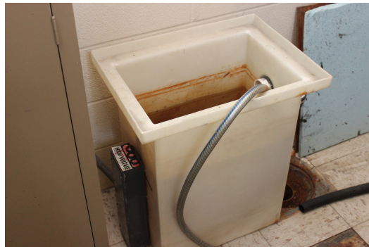
Figure 3.6: Resistor bank cooling setup.
