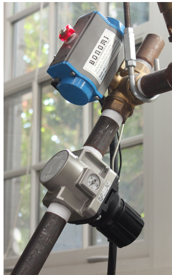
Figure 3.10: Regulator (bottom), and pneumatic three-way valve (top, blue).
