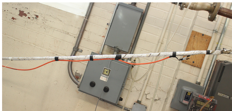
Figure 3.13: Heated sample line.
