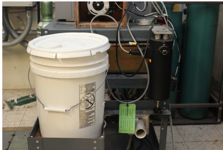
Figure 3.15: Heated filter and chiller.
