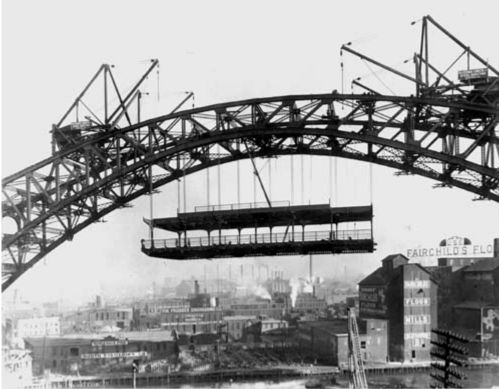
Figure VI. A Section of the Detroit-Superior Bridge put into place by cables and cranes.
