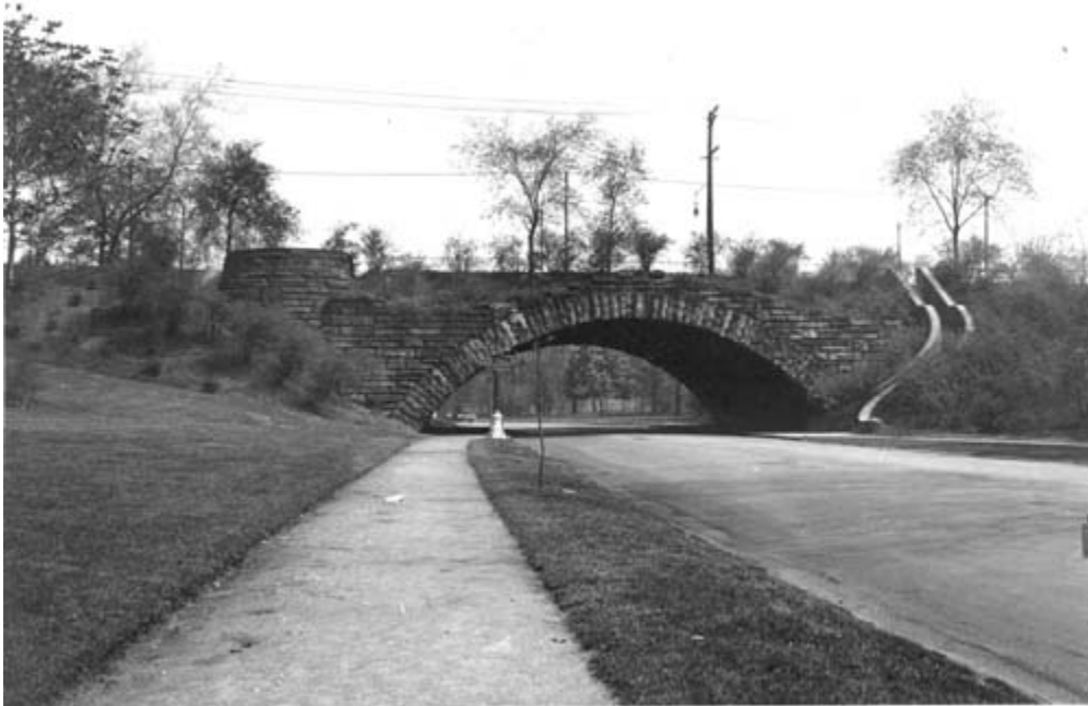
Figure XXI. The Wade Park Bridge over Liberty Boulevard, designed by Charles Schweinfurth in 1900.
