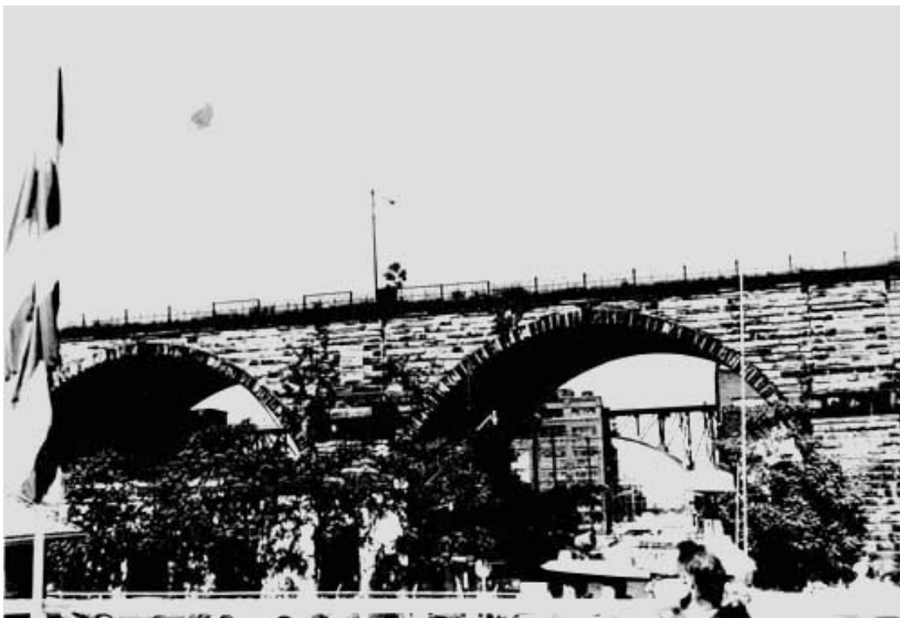
Figure IV. Stone arches of the old Detroit Viaduct, still standing over the Cuyahoga River.
