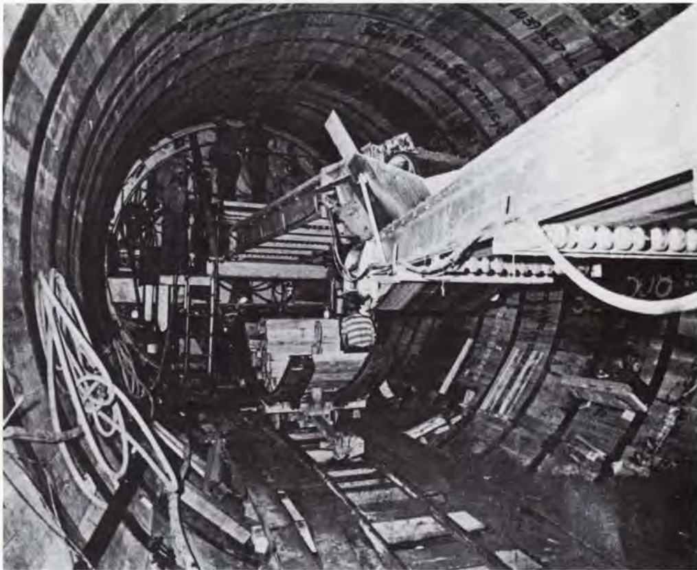
Interior of tunnel under construction, showing barrel-like conventional primary lining consisting of wood lagging braced by steel hoops.
