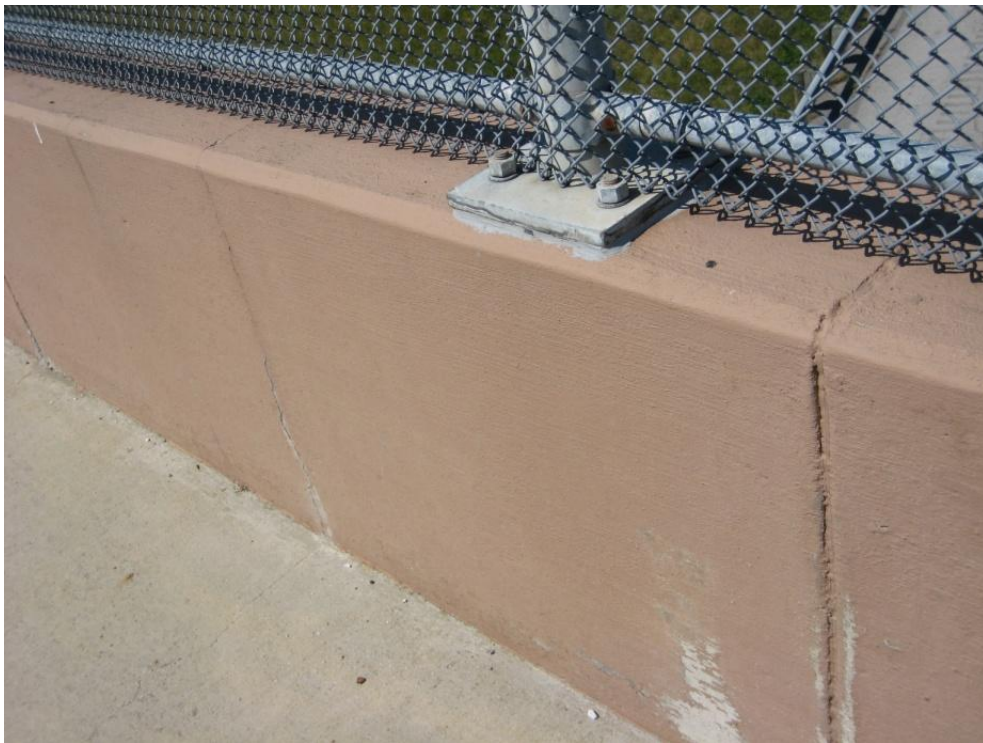
Figure 9: Vertical crack midway between control joints, Canterbury Road
