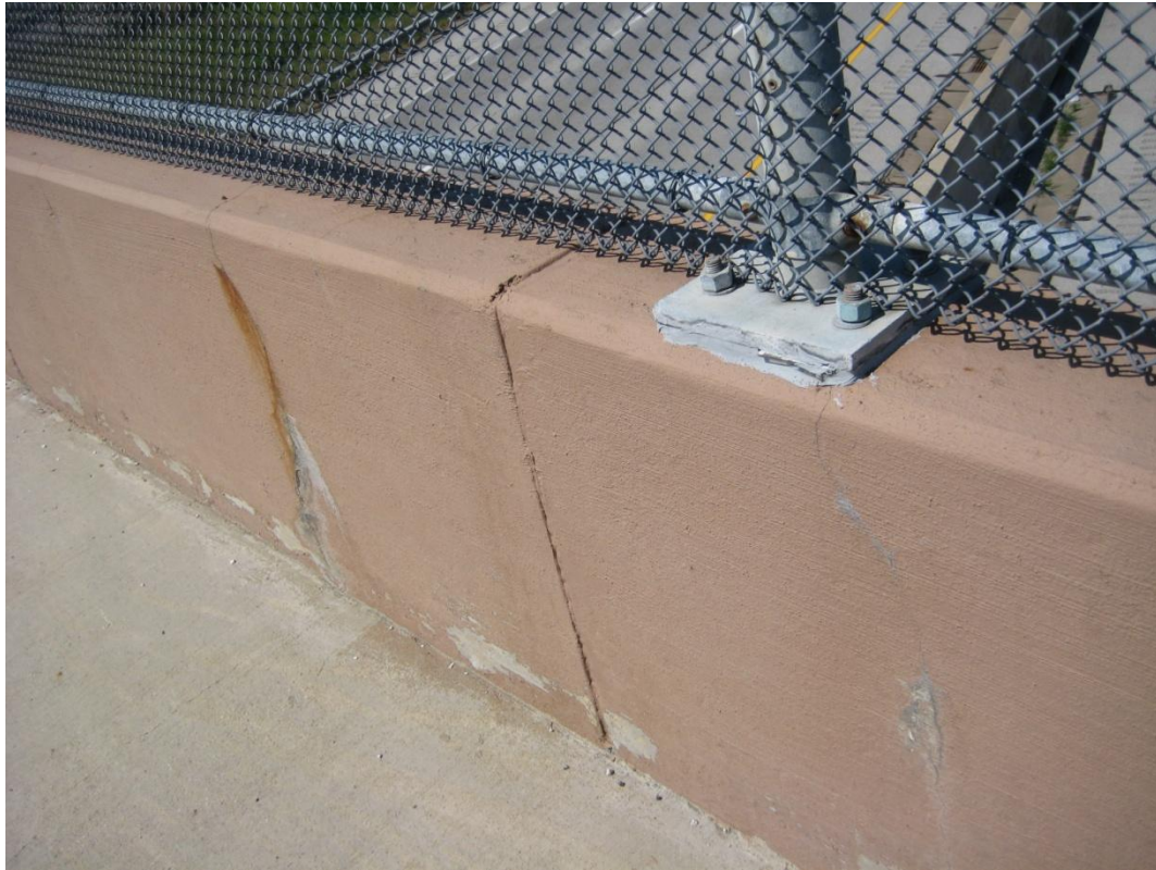
Figure 16: Completely sealed control joint, Canterbury Road
