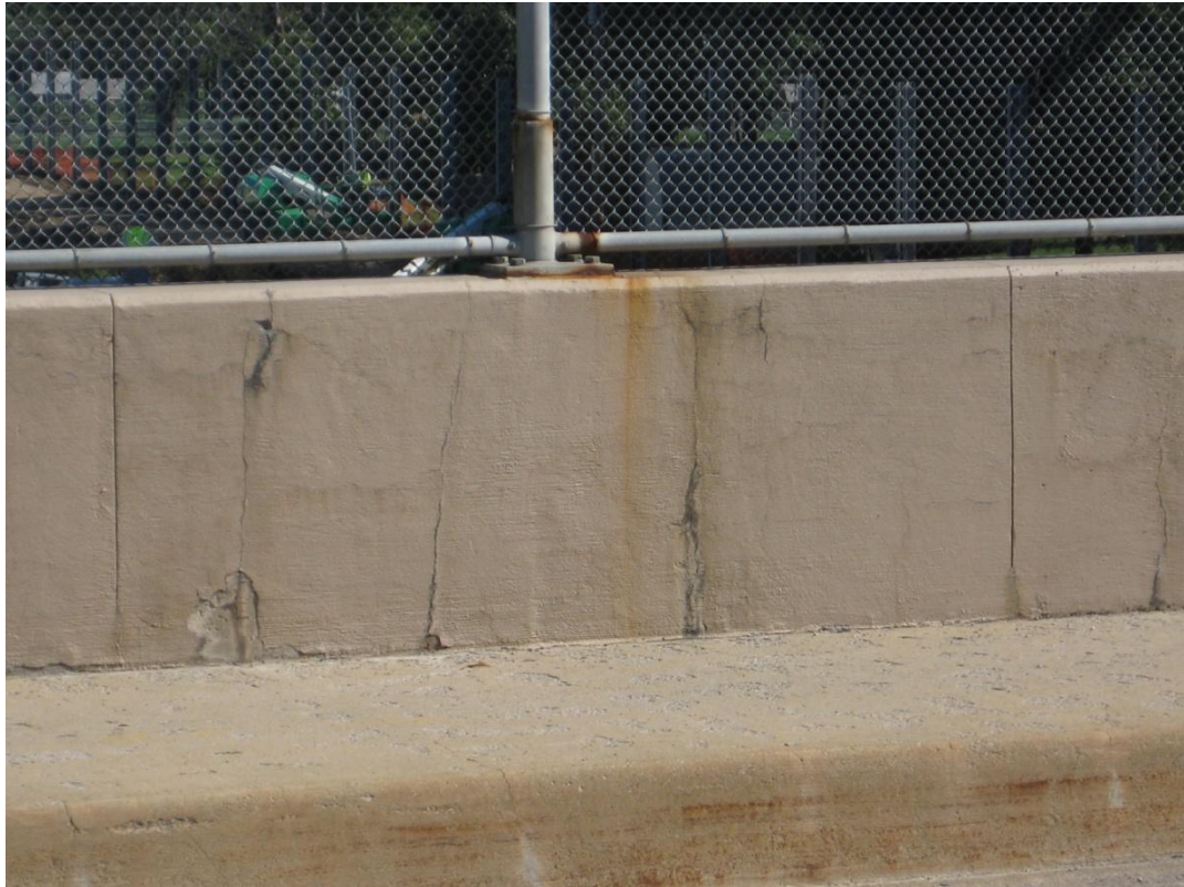
Figure 17: Unsealed control joints with incomplete sawcuts, Sheldon Road
