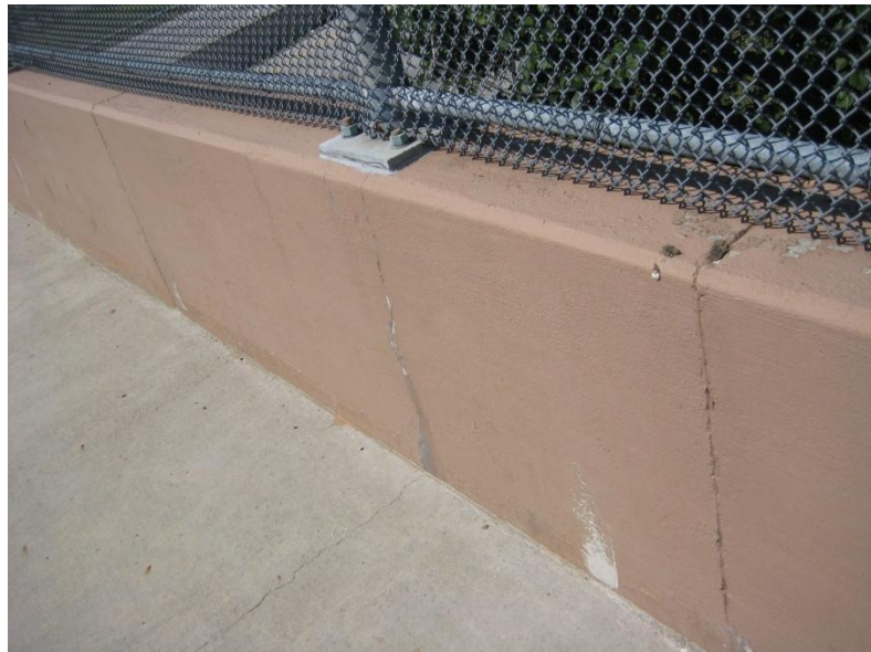
Figure 20: Continuous crack through sidewalk, Canterbury Road
