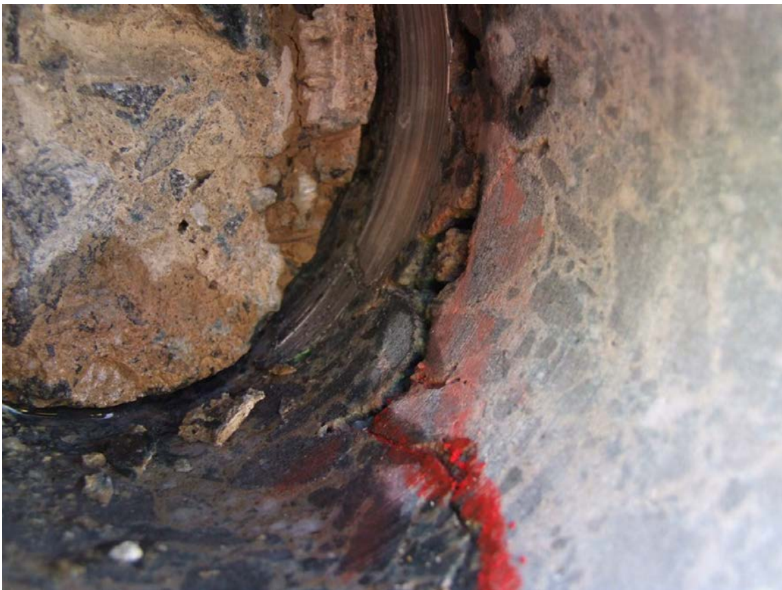
Figure 3: I-95 Parapet Concrete Void (Photo Provided by Fawaz K. Saraf, P.E.)
