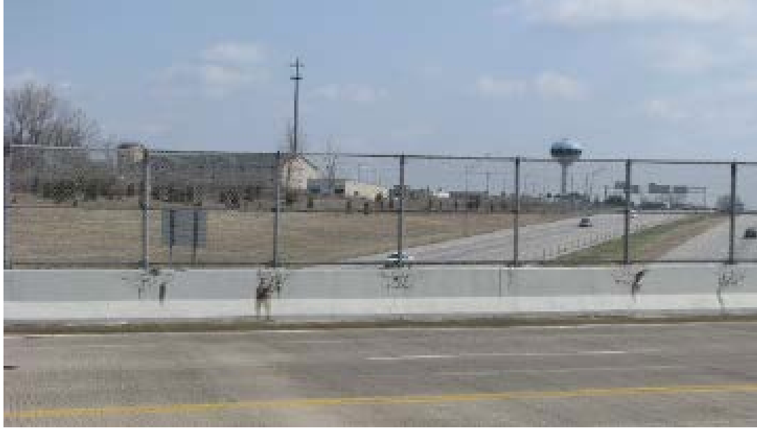
Figure 26: Bridge Number GRE-675-0895 Cracking (Photo Provided by Brandon Collett, PE)
