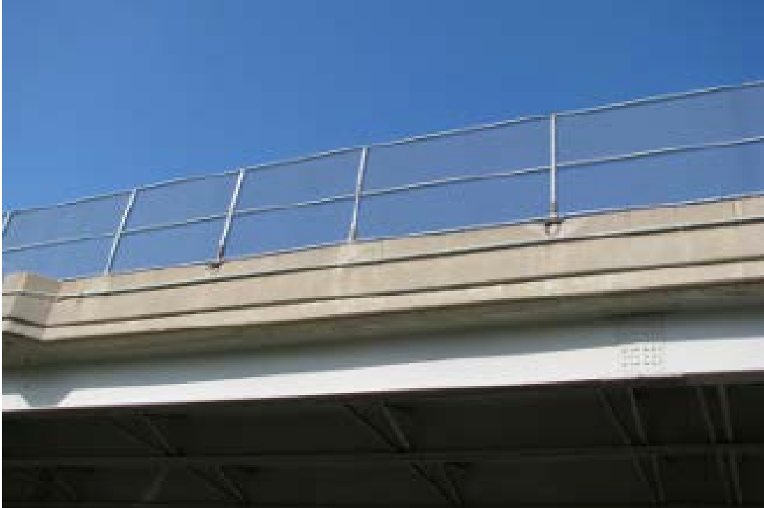
Figure 28: Bridge Number GRE-675-1034 Cracking (Photo Provided by Brandon Collett, PE)
