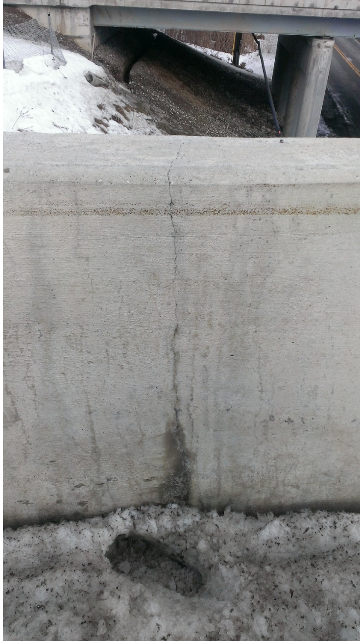
Figure 2: Vertical Parapet Cracking (Photo Provided by Lauren Hedges)
