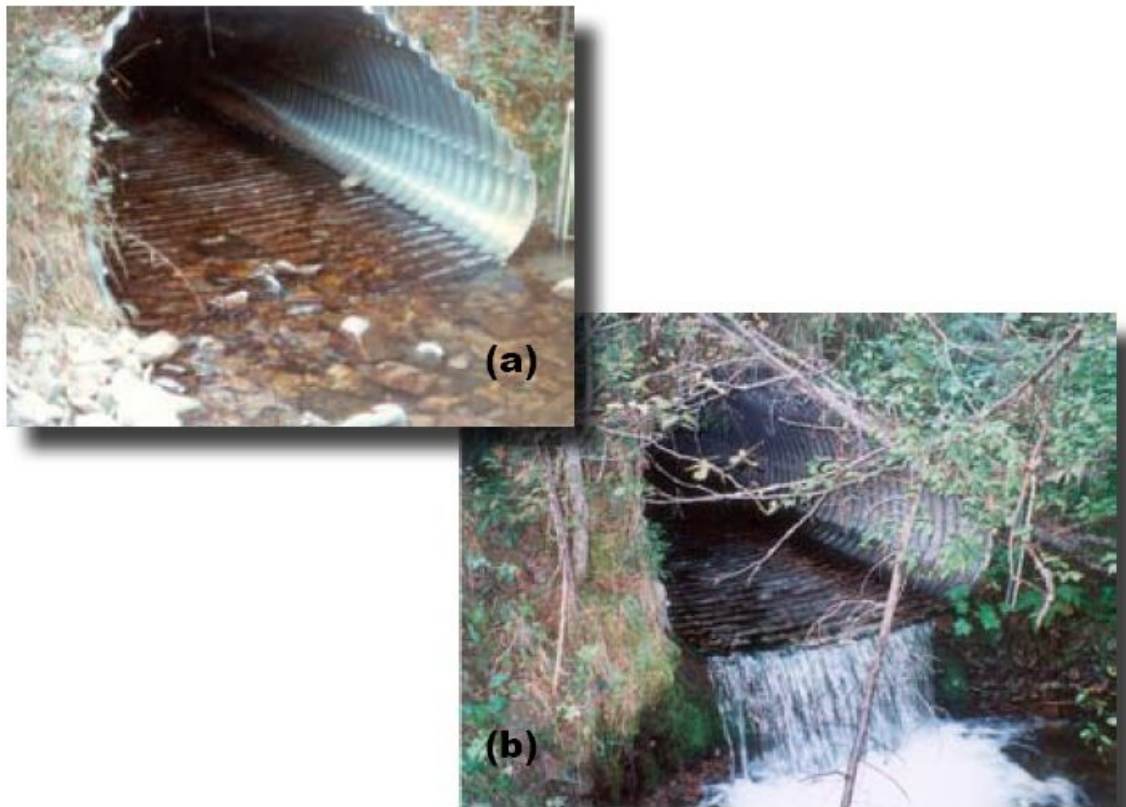
Figure 1.1 Perching of a Culvert as a Result of Long-Term Scouring (Forest Service Stream Simulation Working Group, 2008)
