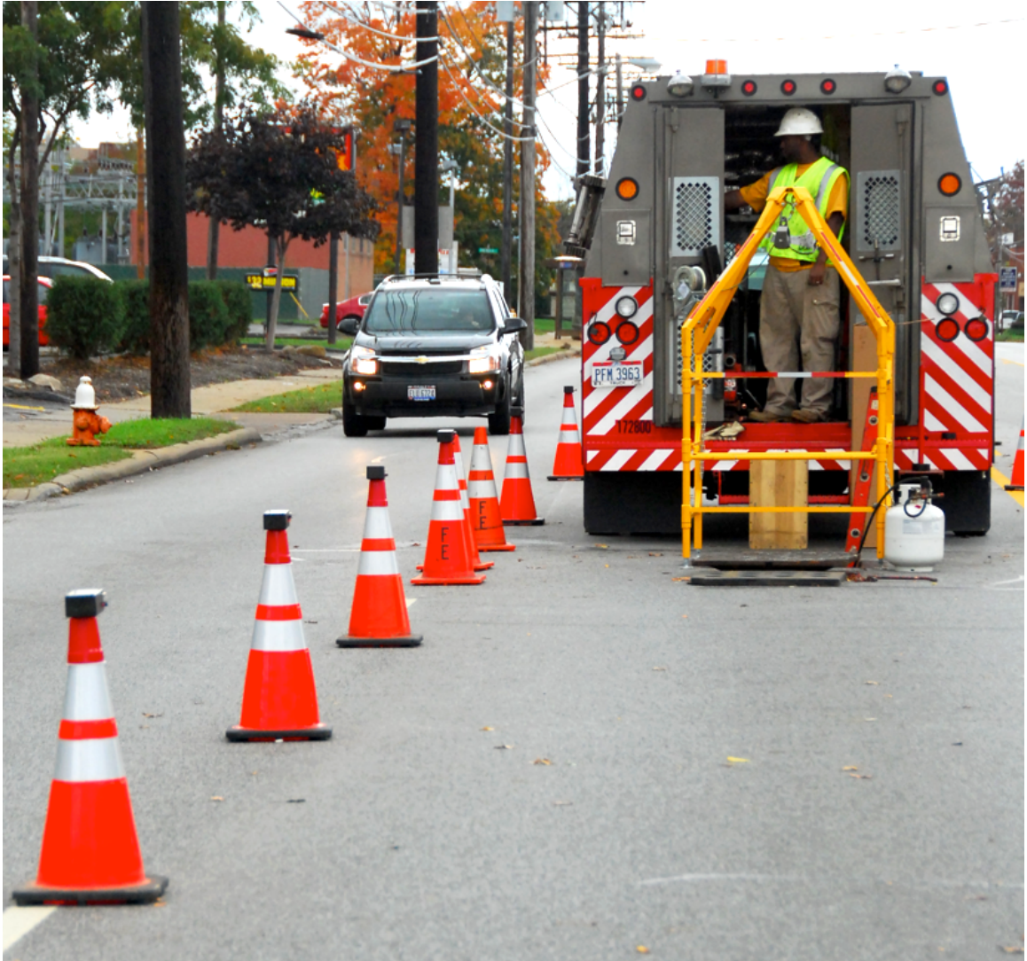
Figure 2: Our sensor net system deployed in a work zone to collect traffic statistics. The sensors are mounted on top of construction safety cones. The placement of the cones is as required by the work zone itself as per the MUTCD, and is not modified by our deployment.
