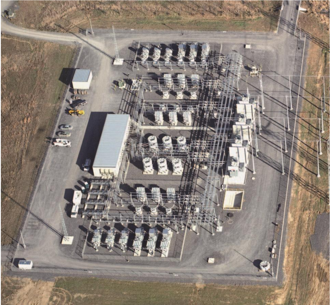
Figure 2: A 500 kV static var compensator, Allegheny power, Black Oak substation, Maryland USA [31]
