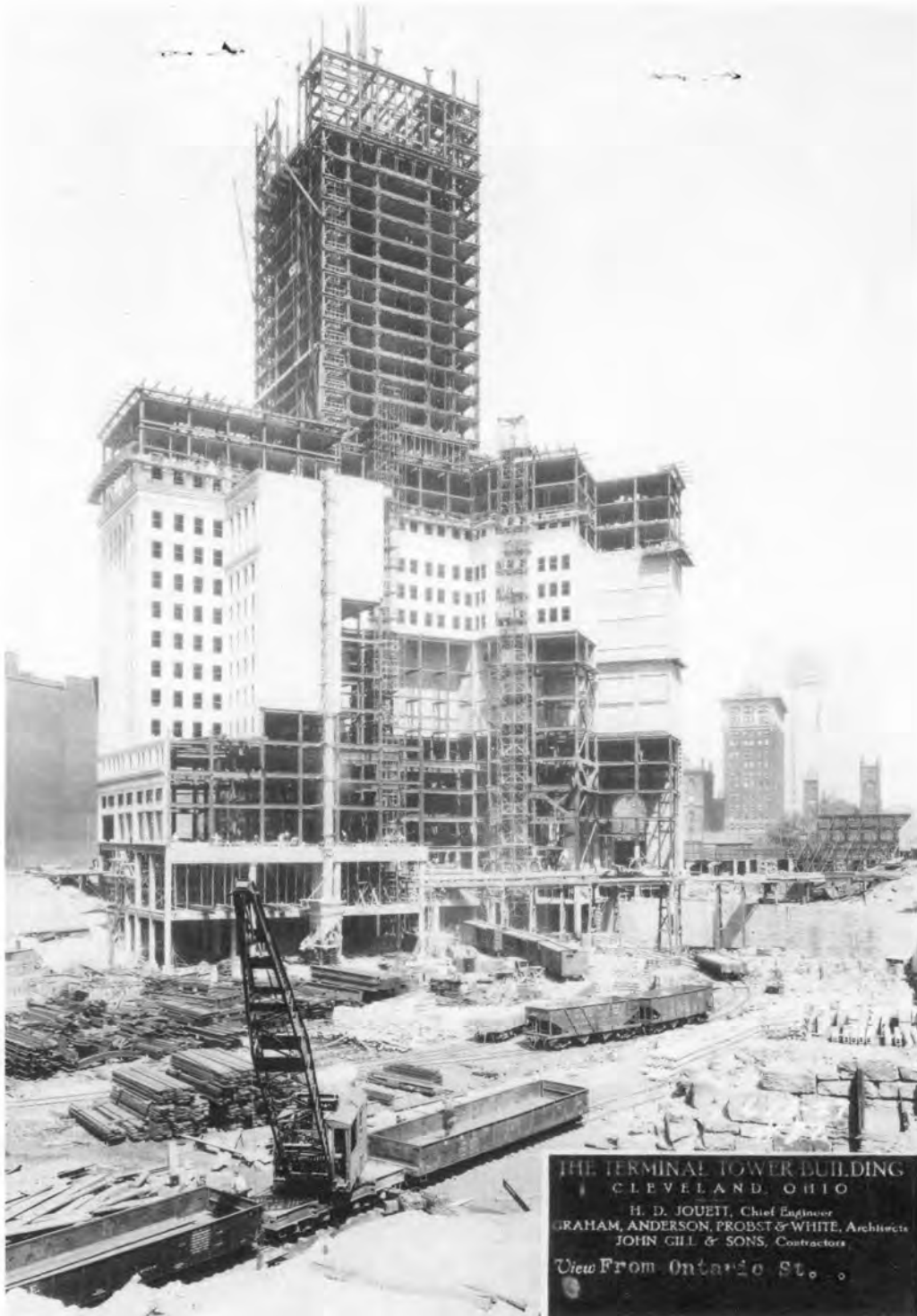
Above: The Terminal Tower under construction. Photograph taken June 13, 1927. Note Old Stone Church in background at right. The story of the building of the Tower begins on page 3.
