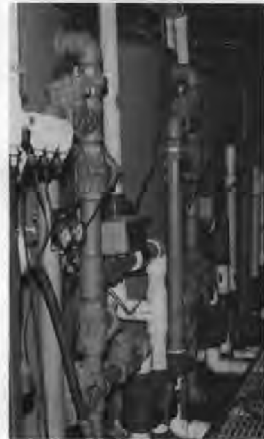
Two carbon filter tanks (foreground) and two depth tanks. They are used to filter "city water" before it is softened and run through the reverse-osmosis-membrane system to produce ultra-pure water for the detector.
