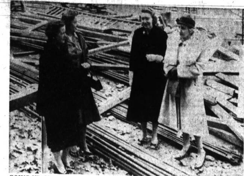
GOING UP: Members of the Mothers' Auxiliary of St. Aloysius Academy, Jersey City, are checking the progress of the three-story addition to the academy. The women are sponsoring a card party-fashion show Nov. 24 at Scheutzen Park, North Bergen, to help pay for the project. Shown above are, left to right: Mrs. Edward Hammill, Mrs. J. Randolph Jones, co-chairman; Mrs. Edward J. Ward, chairman, and Mrs. John E. Ward.
