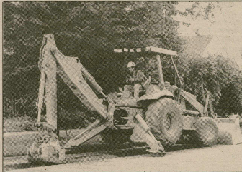
A backhoe digs up Alder Street across from campus this past week. Construction caused discolored water on campus among other problems.
