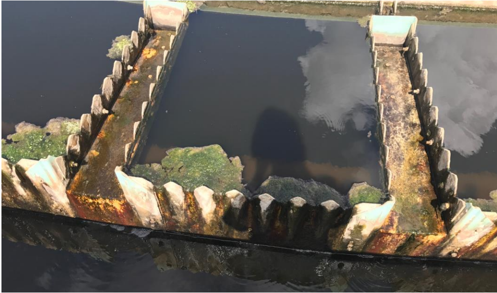
Figure 23. Algae growing in the secondary clarifier.
