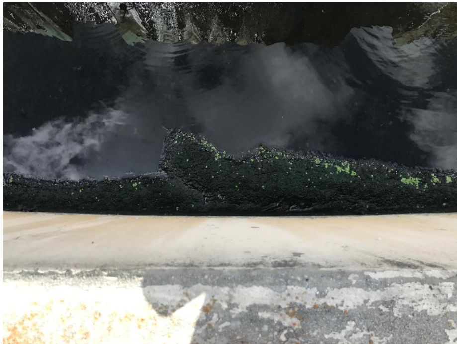
Figure 24. Algae growing over the weir of the secondary clarifier.
