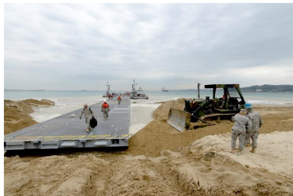
Figure 6. U.S. Soldiers with the 331st Transportation Company install a section of the Trident Pier causeway in preparation for ship-to-shore unloading operations on April 15, 2013, in Pohang, South Korea (Courtesy of U.S. Army).
