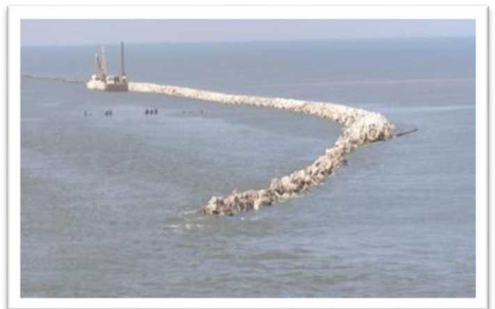
Figure 1-7 Southwest Pass jetty after repair, circa May 2009 - Sep 2010 (source: U. S. Army Corps of Engineers, New Orleans District)
