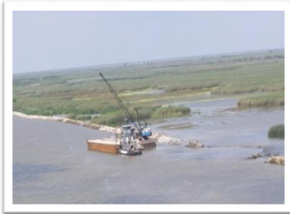
Figure 1-10 Foreshore rock protection damage (source: U. S. Army Corps of Engineers, New Orleans District)
