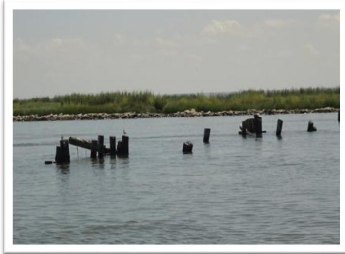
Figure 1-8 A typical timber pile dike before repair (source: U. S. Army Corps of Engineers, New Orleans District)
