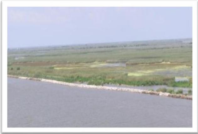
Figure 1-11 Foreshore rock protection after repair (source: U. S. Army Corps of Engineers, New Orleans District)
