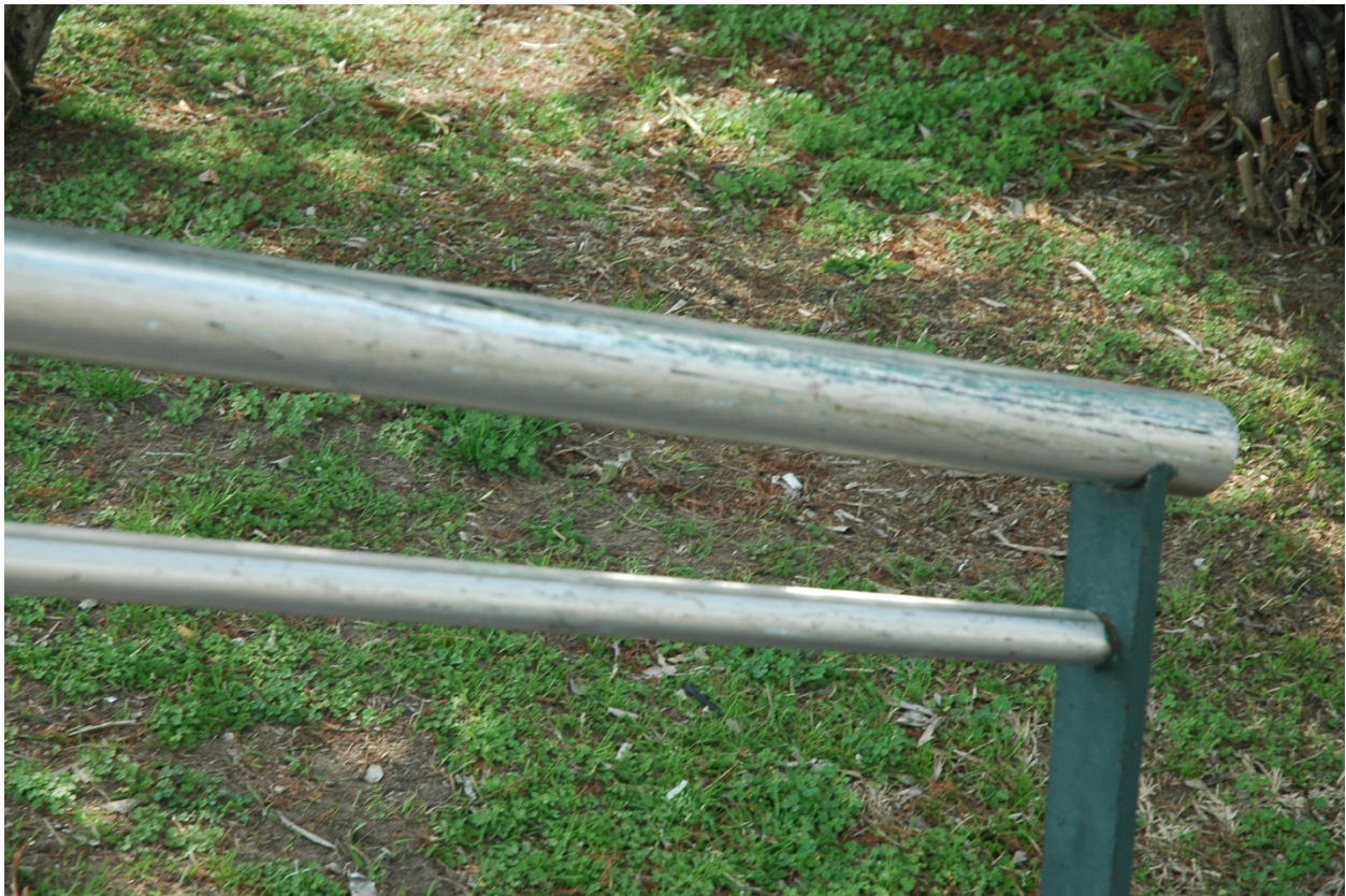
Figure 13. Paint on a stainless steel hand rail is evidence of board slides.
